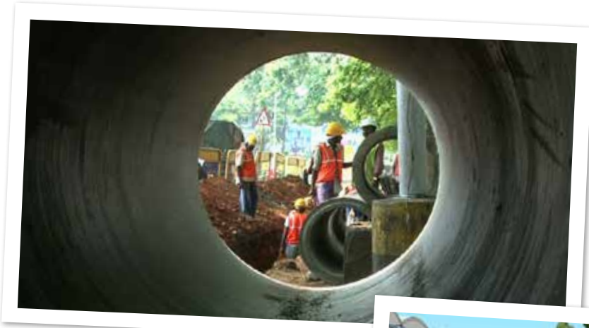
Men at work on a Tender S.U.R.E. road, organizing underground services below the footpath.
